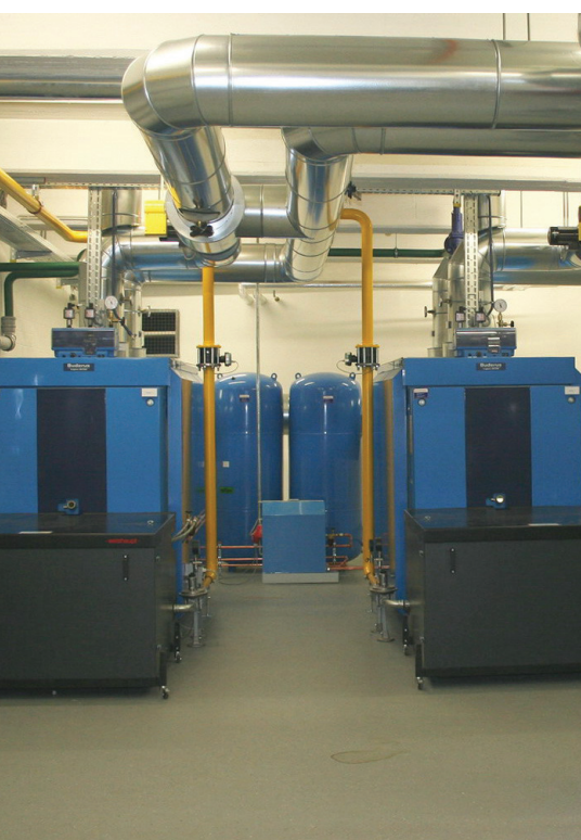
Heizzentrale heating system
